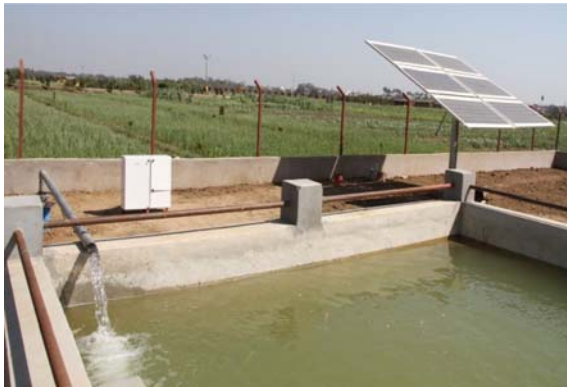
a) Pumping unit for groundwater abstraction into a storage tank
