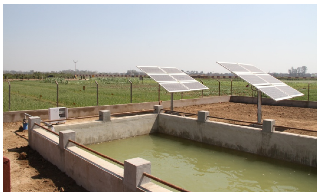
Fig. 1. Solar-powered irrigation pump of the experimental site
